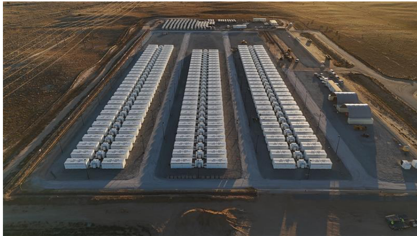
Clēnera's Atrisco Battery Storage Project
